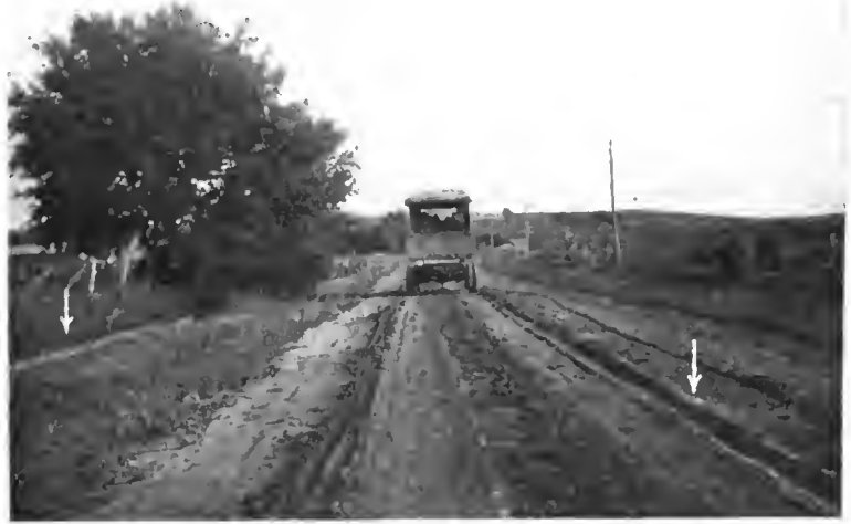
No attempt of any kind of road making; travel alone defines the roadway of two ruts divided by a grass center. In wet weather all the water from the high fields on the right crosses the road to the low fields on the left. The rank growth in the left foreground shows how long the water stands. During wet periods the road is more or less flooded and becomes passable only after long dry periods.
